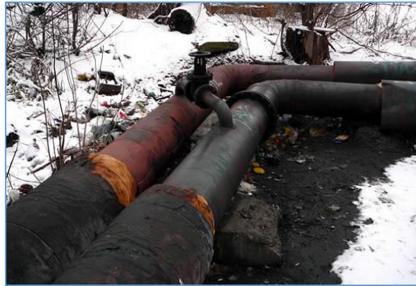
Image 2. Old heating tubes to be renovated by KHURC
